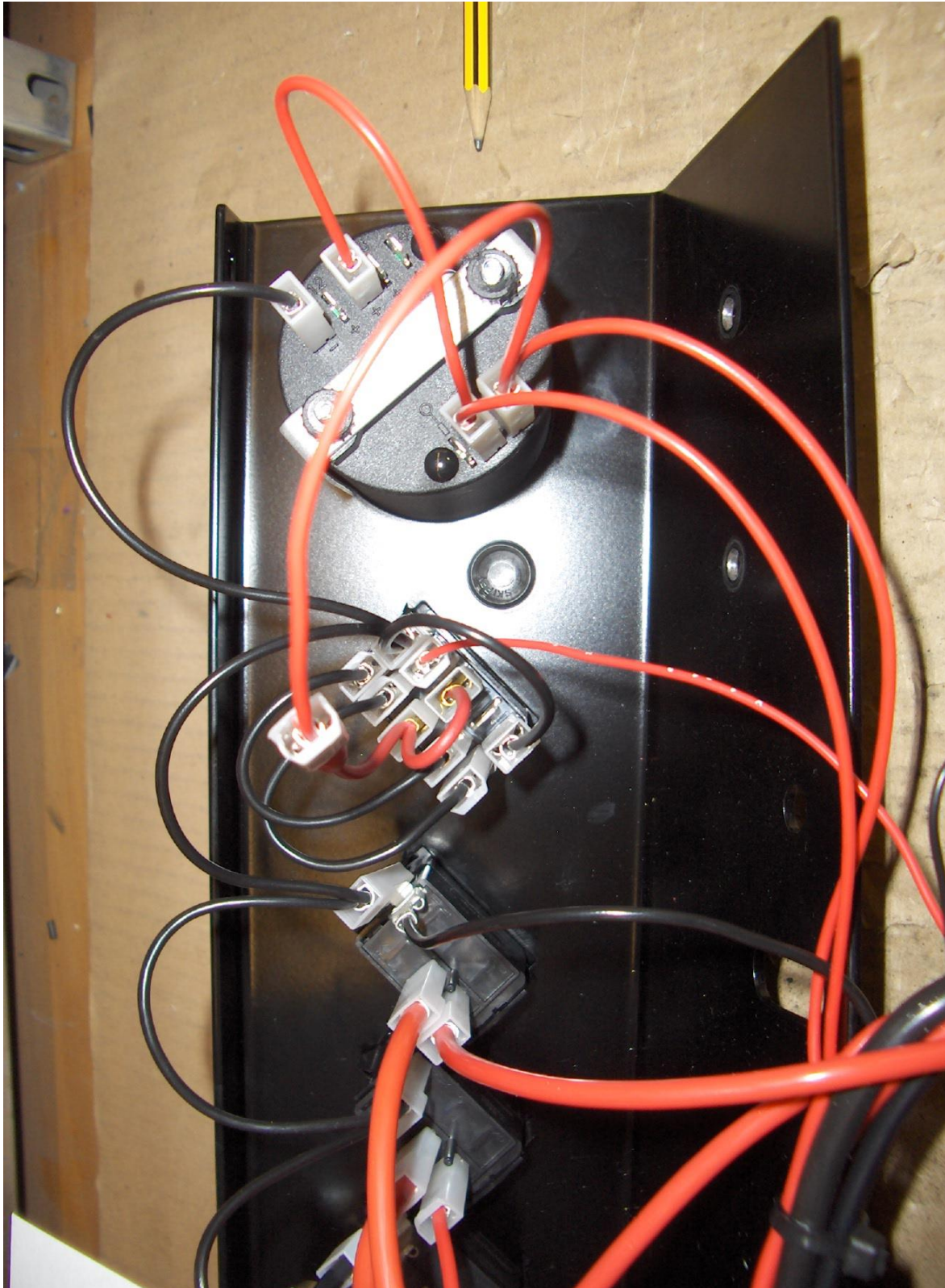
Pic G: Wiring for S-DRIVE-Controller. Blue wire is not needed any more and so is fixed with cable ties directly at the harness.
